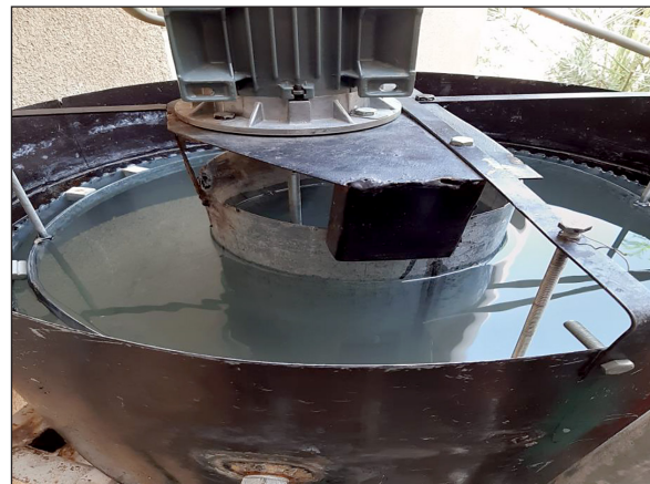
Figure 1. Flash mixing tank
