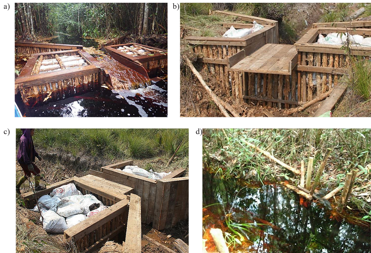
Figure 1. (a) Canal blockage in tropical peat swamp forest at the research location, (b) back view of the canal bulkhead, (c) front view of the canal bulkhead, (d) channel blockage damaged by channel users
