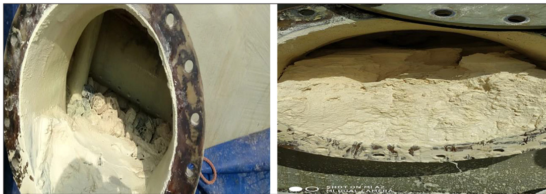
Figure 7. Sulfur deposit in the Tower entry pipe
