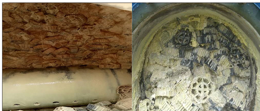
Figure 3. State of desulfurization tower clogging (WWTP Fez : 15-01-2018)
