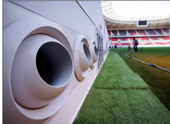
Figure 4. A photo shows the Cold air supply nozzles for open area air conditioning in Qatar. ( https://time.com/6236839/qatar-world-cup-outdoor-air-conditioning-environment/ )
