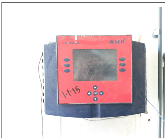
Fig. C-7. JESCO TOPAX DE microprocessor controller (installed January 2015, as marked). The unit provides digital control of chlorine dosing rates, real-time residual monitoring, alarm outputs, and data logging — replacing the manual fixed-rate approach of the pre-upgrade system. The digital interface enables operators to set and maintain precise dosing targets.
