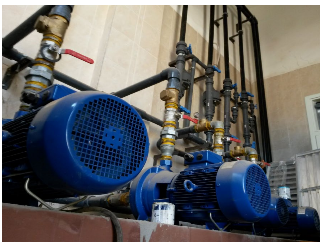
Fig. C-14. Close-up of alum dosing pump motors (blue) showing the robust industrial electric motor specification. Brass flanged connections (yellow-sealed) connect the pump outlet to the stainless-steel injection assemblies. The red ball-valve serves as a manual isolation point for individual pump maintenance without system shutdown.
