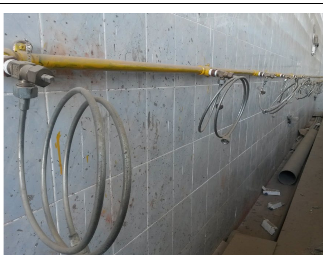
Fig. C-6. Yellow Cl 2 gas supply header running along the chlorination room wall, with individual armoured flexible connections to each gas cylinder. The vacuum-regulated design ensures that any pipe failure causes gas flow to stop automatically, providing a critical safety upgrade over the previous direct-pressure system.
