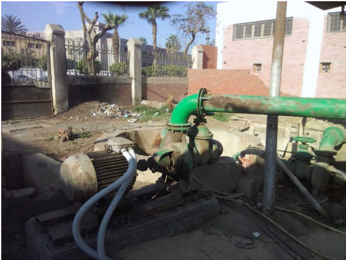
Figure I-3. Pre-upgrade centrifugal pump manifold arrangement at the El-Galaa WTP pump station. The photograph shows the deteriorated condition of the pump housings, discharge manifolds, and associated pipework prior to the 2019 rehabilitation programme (Field survey, 2018).
