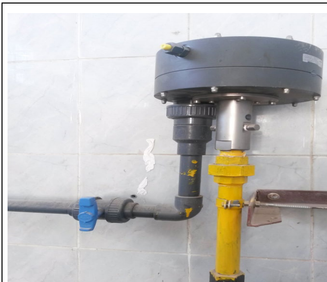
Fig. C-3. JESCO vacuum-operated Cl 2 gas regulator (grey cast housing, upper unit) connected to yellow gas supply pipe via stainless steel injector body. PVC isolating valve (blue handle) controls solution feed line. This unit regulates gas flow and converts pressurized Cl 2 to a safe vacuum-operated dosing stream.
