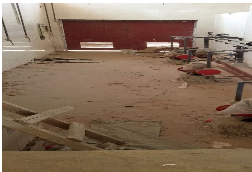
Fig. C-17. Interior of the new chemical dosing building (chlorination and alum rooms), showing tiled walls, ventilation windows, and chlorine detection sensor (ceiling-mounted, upper left). The purpose-built facility meets occupational safety requirements for chemical handling, replacing makeshift pre-upgrade arrangements.
