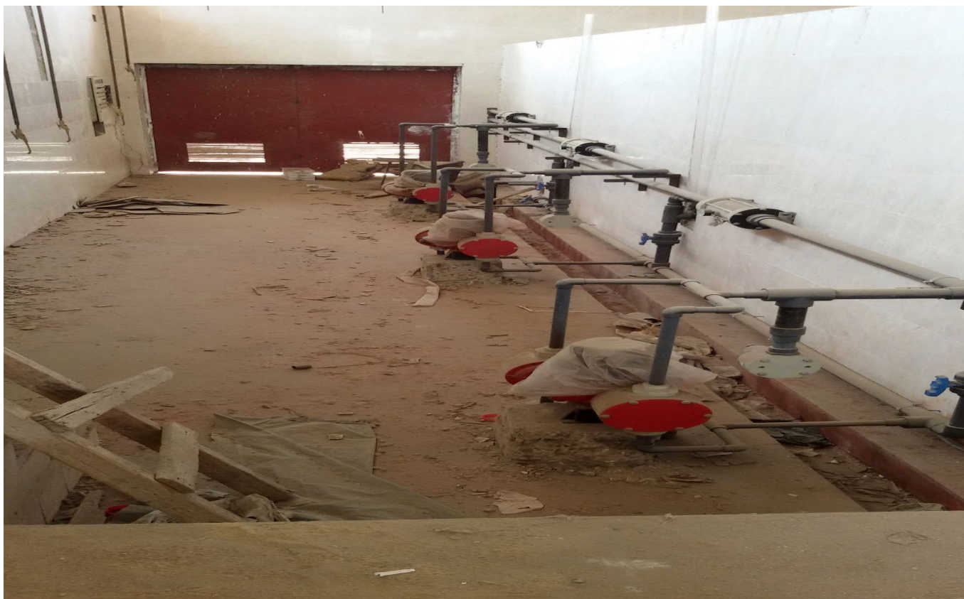
Fig. C-11. Alum dosing pump station during construction phase (June 2015), showing five chemical dosing pumps (red end-caps, still covered in protective wrapping) mounted on individual concrete plinths along the pump room wall. The PVC distribution manifold headers are already installed on the wall brackets (grey pipes). The building is in active construction — earthen floor, construction materials present — documenting the transition from manual dry-feed to automated pump-driven dosing that enabled the post-upgrade alum dose reduction from >60 mg/L to ~35 mg/L.
