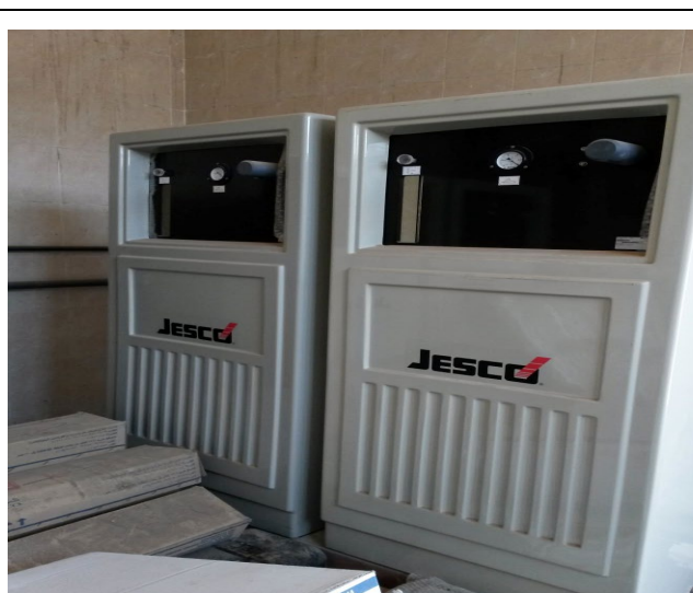
Fig. C-10. Side-profile view of the JESCO chlorinator cabinets showing the ribbed fiberglass housing designed for corrosion resistance in chlorine environments. Pressure gauges (top of each unit) monitor gas supply pressure continuously. The sealed cabinet design significantly reduces personnel exposure to Cl 2 fumes compared to the open cylinder-and-regulator arrangement previously in use.
