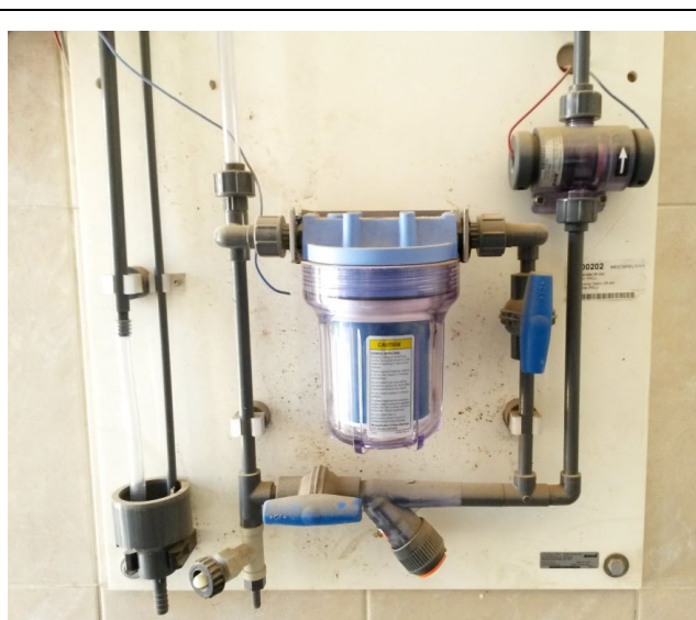
Fig. C-8. JESCO TOPAX DE controller (left) with associated sample water station (right panel). The station includes a sediment pre-filter (blue transparent housing), flow indicator, electrode holder for amperometric Cl 2 sensor, and automated flow-control valve. This enables continuous real-time measurement of treated water Cl 2 residual as the feedback signal for the TOPAX DE controller.
