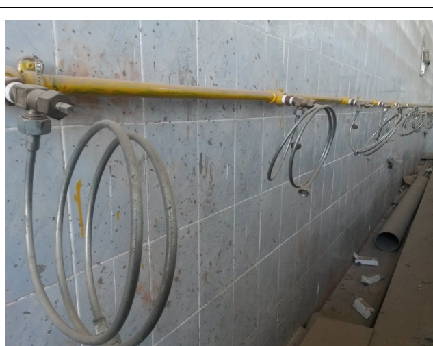
Fig. C-2. Pre-upgrade chlorine gas distribution manifold (yellow pipeline) with flexible armoured hoses connecting individual Cl 2 cylinders to the chlorinator unit. Each hose serves one cylinder in a multi-cylinder bank configuration.
