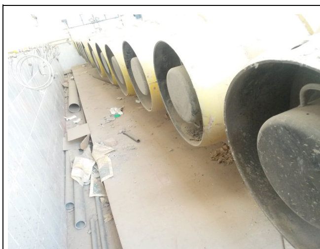
Fig. C-1. Pre-upgrade Cl 2 gas cylinders stored at El-Galaa WTP. Multiple large-capacity pressurized steel cylinders (yellow painted) awaiting decommissioning during the upgrading works, June 2015.
