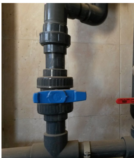
Fig. C-16. Detail of PVC dosing line showing blue ball valve (isolation), stainless-steel pressure gauge (0–250 kPa range), and red ball valve (fine control/sampling). The chemical-resistant PVC piping throughout the alum and chlorine dosing rooms eliminates the corrosion problems that affected the pre-upgrade metallic infrastructure, reducing maintenance requirements.
