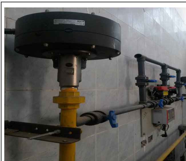
Fig. C-5. Overview of JESCO chlorine dosing system installation showing vacuum regulator (left, grey/yellow), solution distribution pipework in PVC (grey), isolation valves (blue handles), motorized actuator (red), and wall-mounted control panel. The yellow pipe carries Cl 2 gas under vacuum from the cylinder bank to the regulators.
