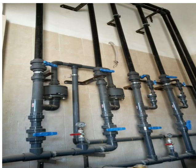
Fig. C-15. PVC injection manifold for the alum dosing system showing four parallel dosing lines, each equipped with: an inline check valve (cylindrical body with red indicator), a blue ball isolation valve, a pressure gauge, and a red manual shut-off valve. This manifold configuration prevents backflow of raw water into the chemical dosing lines and enables independent line isolation.
