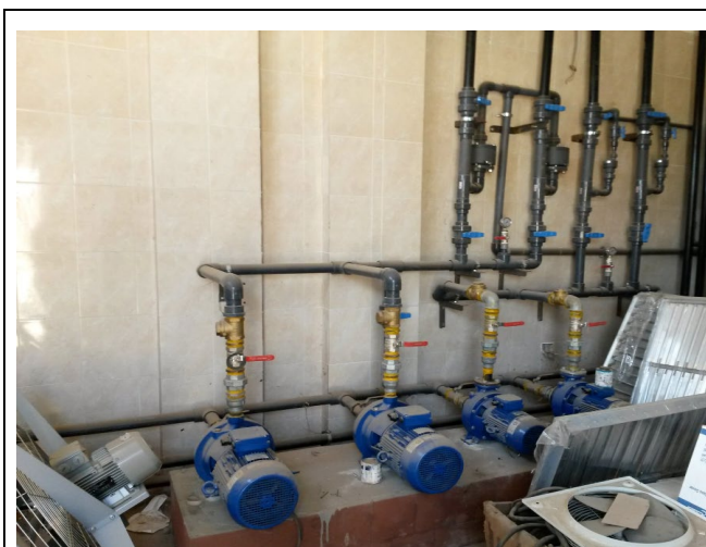
Fig. C-12. New alum dosing pump station (operational) showing four blue electric motor-driven centrifugal pumps mounted on a reinforced concrete plinth, with individual PVC discharge piping, brass isolating valves (yellow seals), and pressure gauges. The four-pump configuration (3 duty + 1 standby) provides full operational redundancy and enables independent dose adjustment to each clarification unit.
