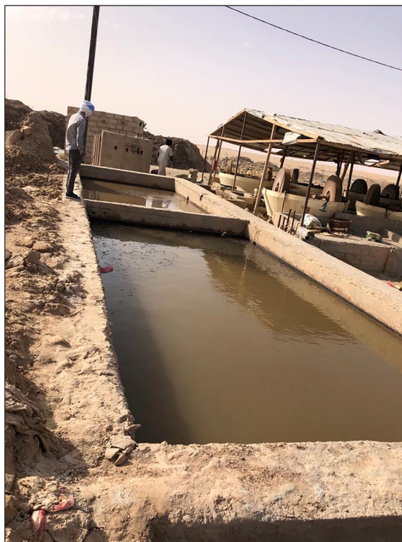
Fig. 3. Photos showing the process water basins in the treatment center
