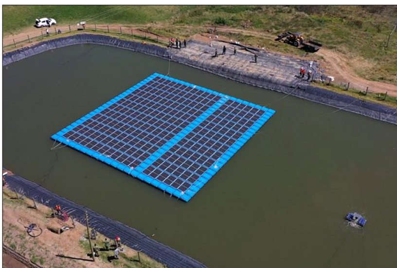
Figure 2. Pilot project of 69 kWp FPV in Naivasha, Kenya [27]
