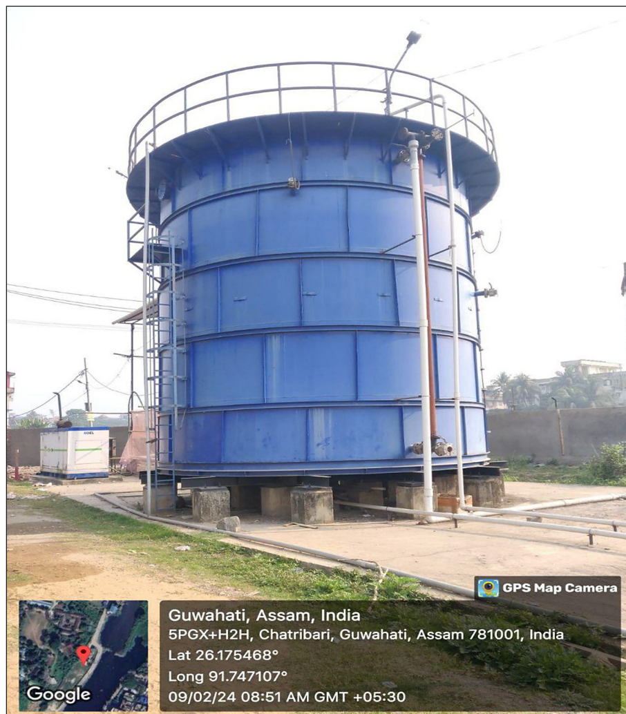
Figure 9. Bio-methanation plant, Chatribari
