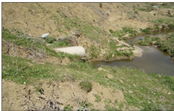
Figure 10. Direct discharge of excess stormwater into the Bougheoul wadi at the urban fringe, documenting the unregulated outfall configuration of the combined sewer network. Source: DRE (2021)
