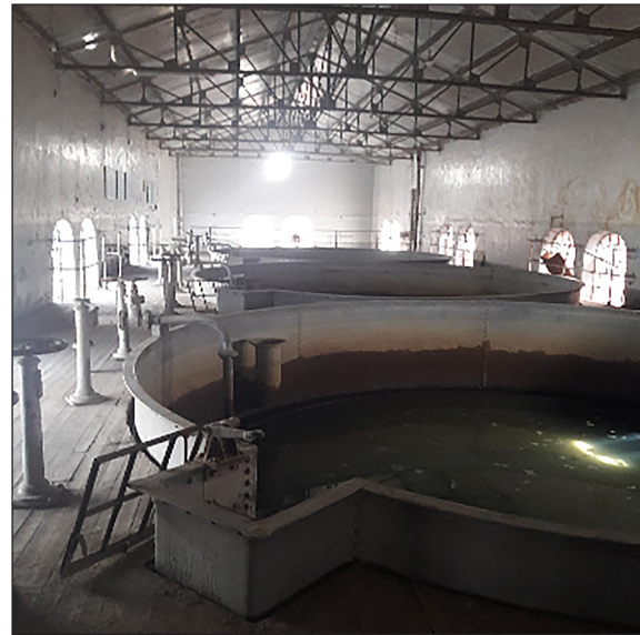
Figure 4. Rapid sand filter building prior to rehabilitation, showing the six circular metallic filter vessels originally commissioned in the early twentieth century. The deteriorated condition of the units is evident from visible surface corrosion on the filter vessels and the absence of dedicated backwash pumping infrastructure, reflecting decades of near-continuous operation without major structural refurbishment
