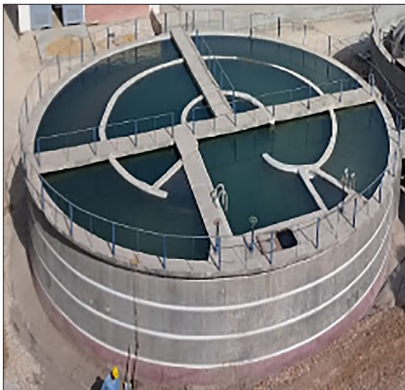
Figure 3. Representative clari-flocculation unit prior to upgrading, showing the central flocculation zone and surrounding settling annulus
