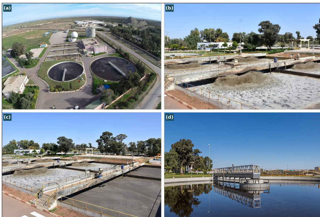
Figure 2. Views of the Khouribga WWTP: (a) overall aerial view, showing the two circular clarifiers, the aeration basins, the digester (white dome) and the storage silo, with an OCP Group phosphate-tailings pile in the background; (b) and (c) biological aeration basins in operation, showing mixing/aeration of the mixed liquor; (d) secondary clarifier with scraper bridge and digester in the background.
